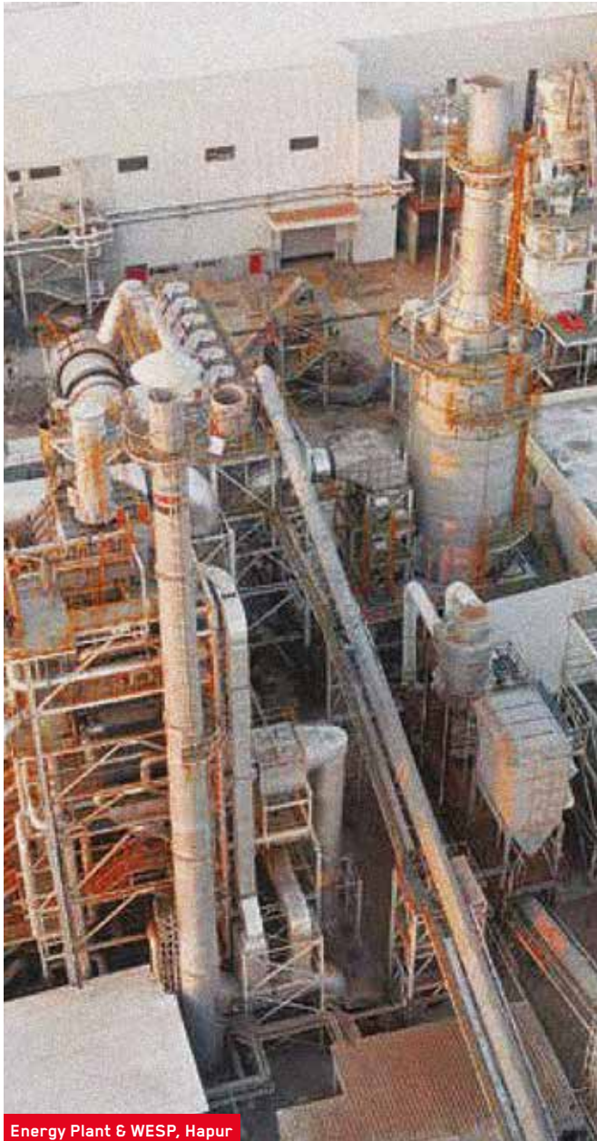
Energy Plant & WESP, Hapur
