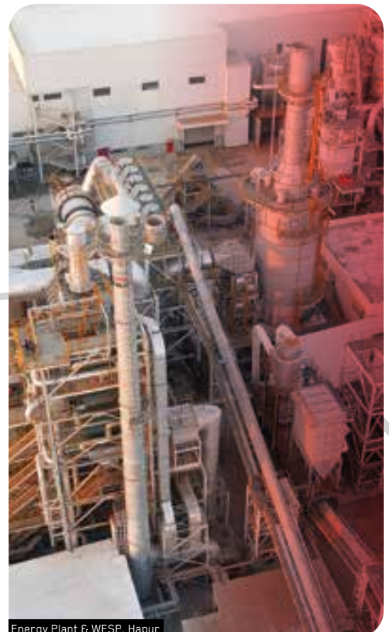
Energy Plant & WESP, Hapur
