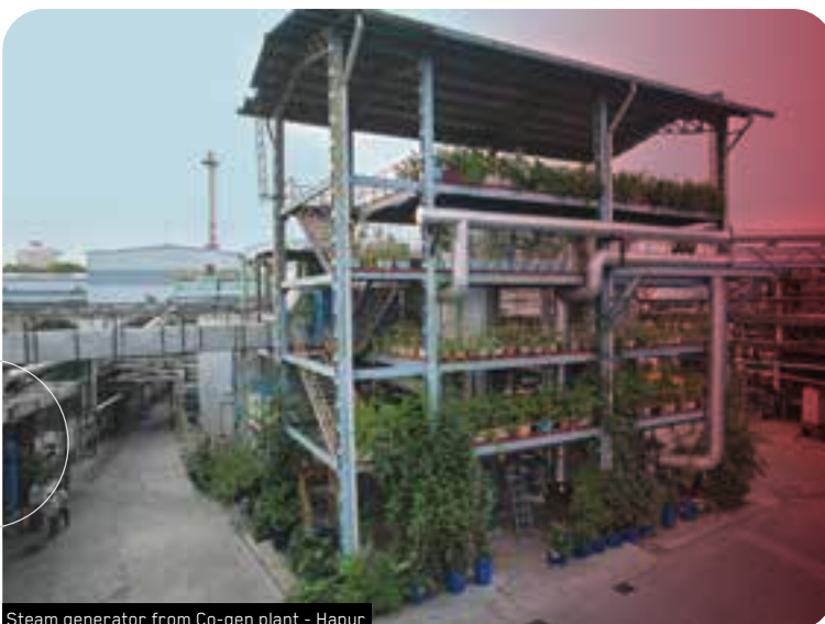
Steam generator from Co-gen plant - Hapur
