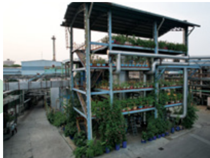
Steam Generator from Co-Gen Plant-Hapur
