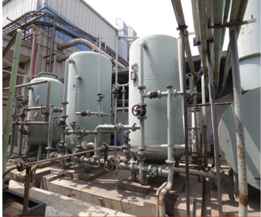
RO Filtration System, MIL Hapur
