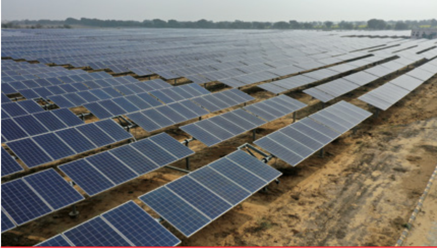
5 MW Ground Mounted Solar Power of Merino Industries- Rohad (in Haryana)
