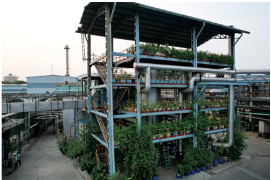
Steam Generator from Co-Gen plant-Hapur
